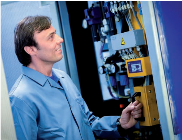
Preventive on-site maintenance service
